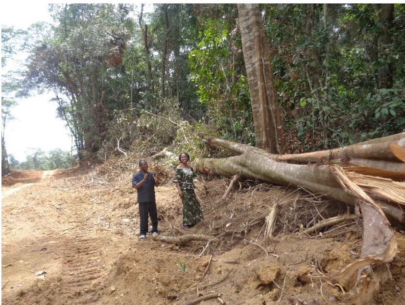
Illustration 1: Bishop and Sister Innis on the newly bulldozed John Dean Town Road
